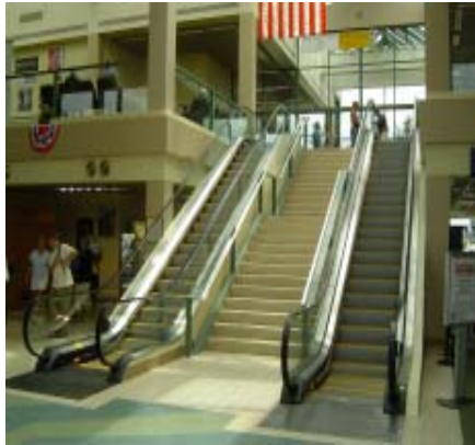
The escalator installation project was completed this past June and provides easier access to the upper level for RFD passengers.
